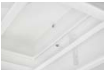
Pressure measurement point, detail
